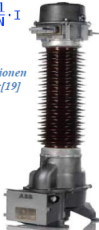
Figure 15- Current transformer on 130 KV side
